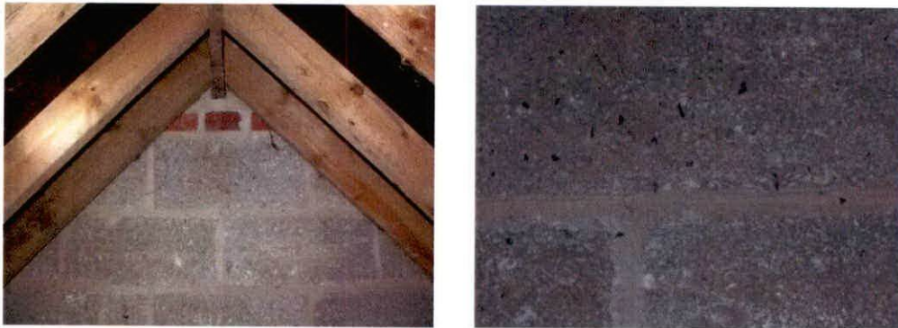
Figs. 17 & 18 Lightly cobwebbed gable with bat droppings on the gable wall
